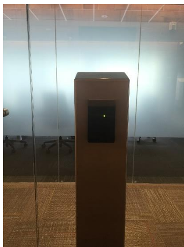
Figure 1 Access Control Door Card Reader
