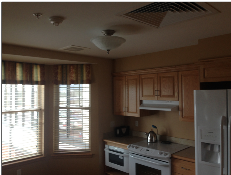
A smoke detector was installed in this kitchen. At the final inspection it was replaced to prevent unwanted alarms.
