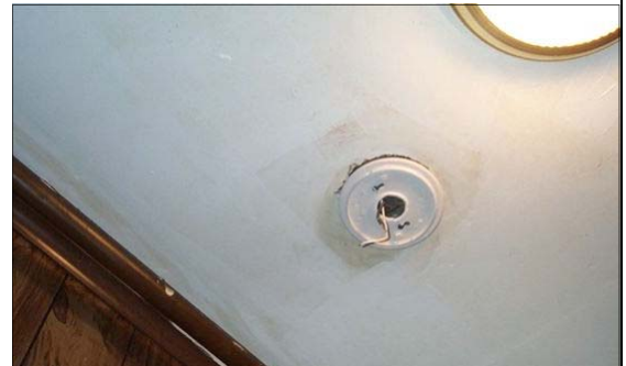
MISSING SMOKE ALARM
