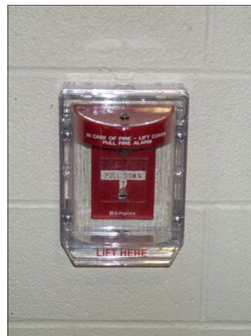
A PROTECTED PULL STATION
