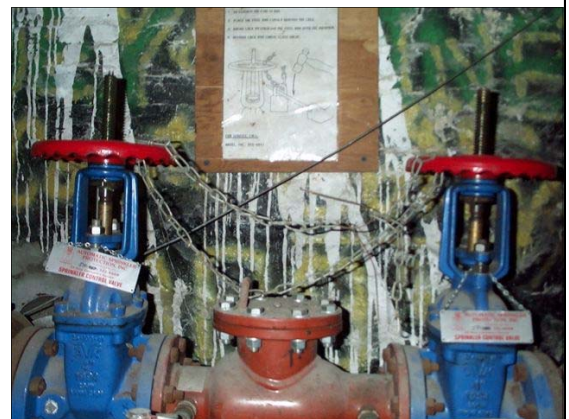
SPRINKLER VALVE ON
