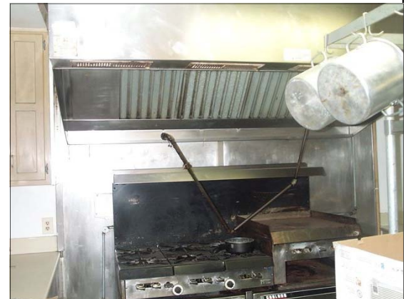
DAMAGED HOOD SYSTEM
