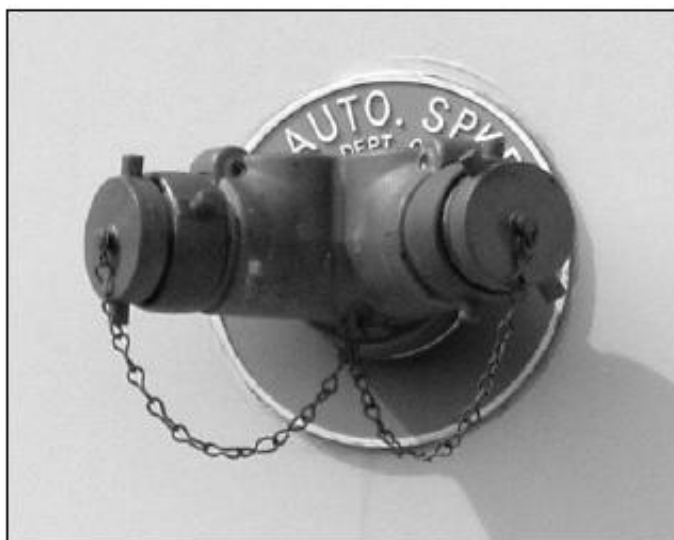
Figure 912.4 FIRE DEPARTMENT CONNECTION WITH SIGN
