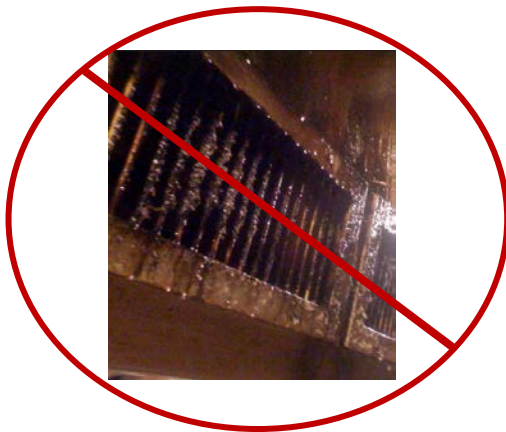
Figure 4: Unacceptable amount of grease Plate
