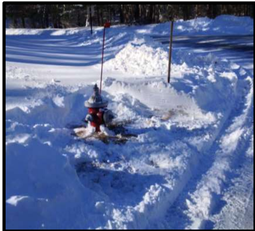
FIGURE 3: Cleared Hydrant with Flag
