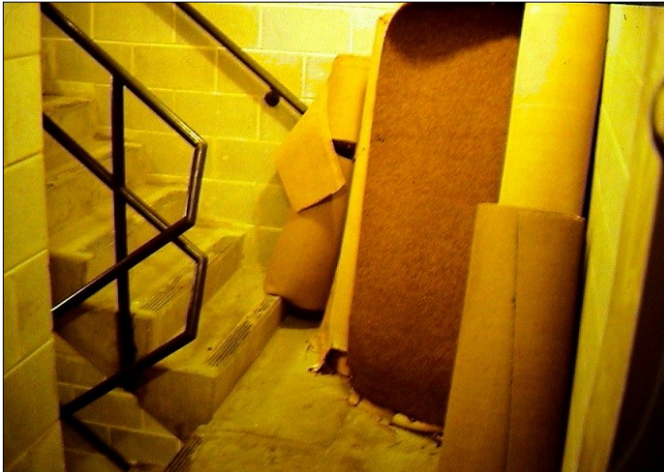
Exhibit 6. Rolled carpet stored in an exit enclosure. (Photo courtesy of Jake Pauls)
