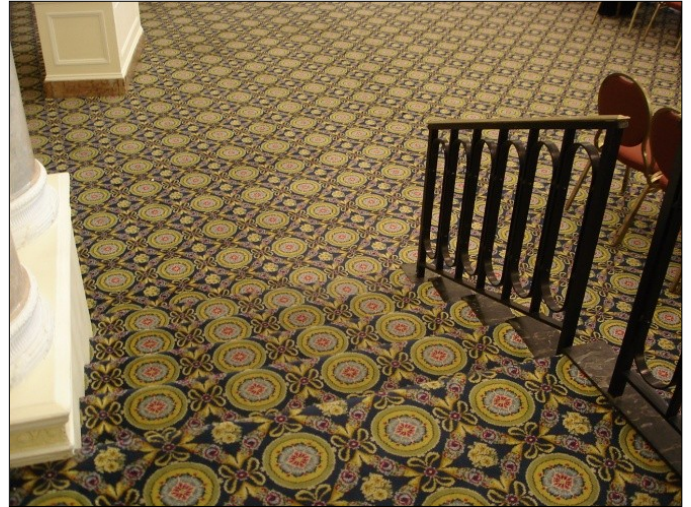
Exhibit 4. Patterned carpet obscures any indication of tread edge location. (Photo courtesy of Jake Pauls)
